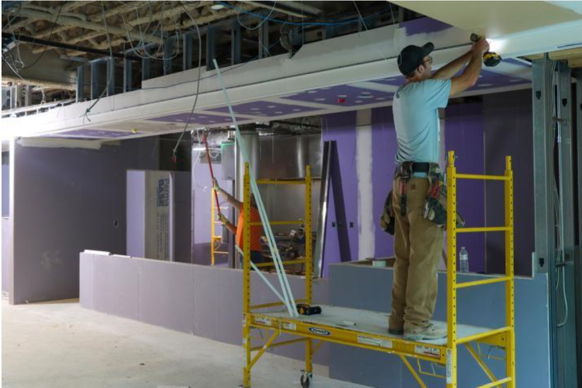
Construction crews continue renovation work at Glenville State University in the Mollohan Campus Community Center snack bar area.
