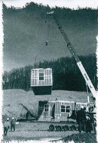
A second story module is gently lifted into place. (Pioneer Village Photos Courtesy of Joe Wilmoth.)
