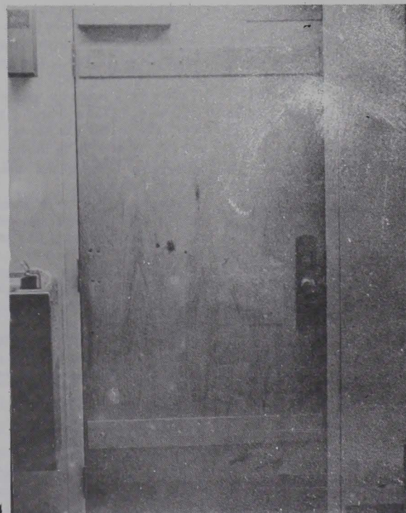
This door on 6th floor has been damaged beyond repair. Note the holes and the steel plates hiding drilled "peep" holes. This is one of the many unfortunate results of the vandalism on the GSC campus this year.
